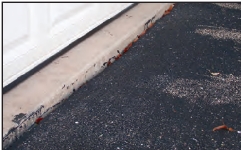
Settlement at garage threshold
