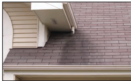
Downspout discharge directly onto shingles
