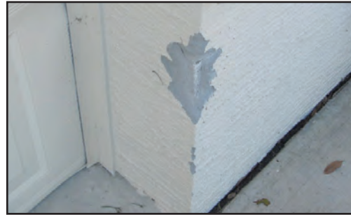
Damage near garage
