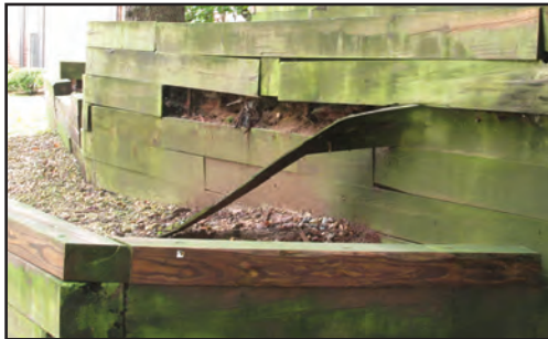
Wood rot and wall deflection
