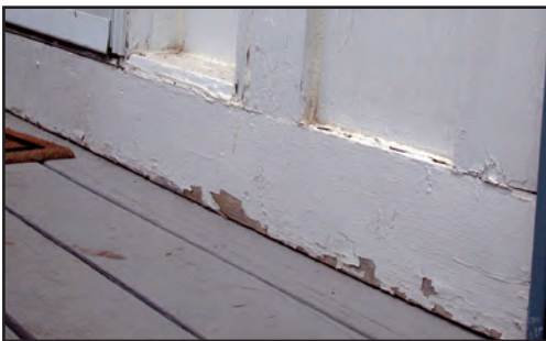
Paint finish deterioration
