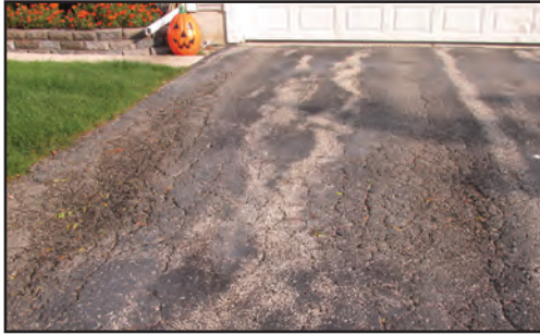
Tire ruts, deterioration and cracks at unit driveway
