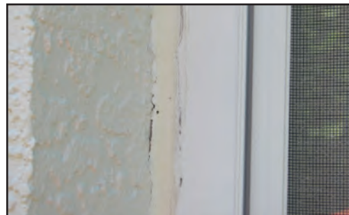
Sealant adhesion failure
