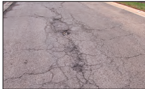
Cracks and potholes
